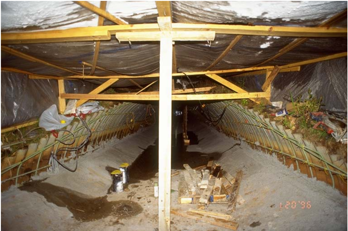
Invert concrete and arch rebar in place with winter snow shelter overhead
